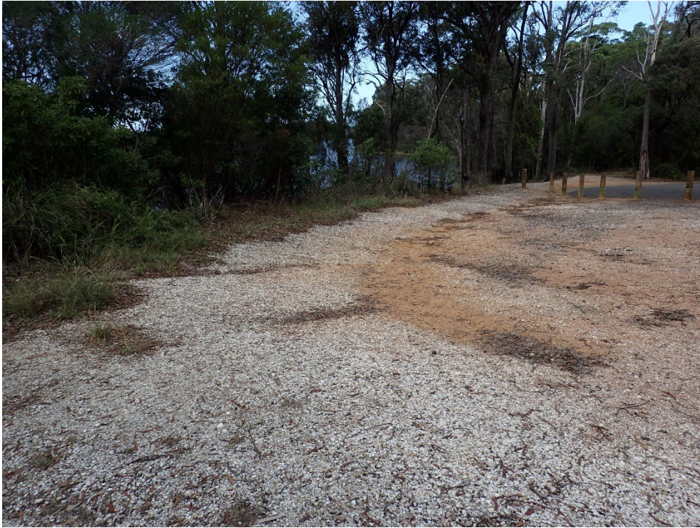
Figure 4: Eroding surface of former vehicle turning area, Fairhaven Point Way
