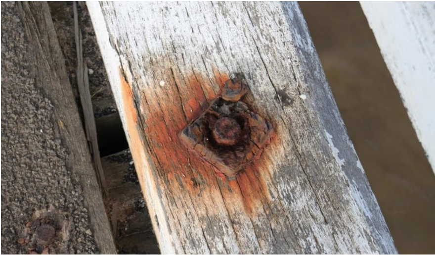
Rusting fixings holding down kerbs, June 2021
