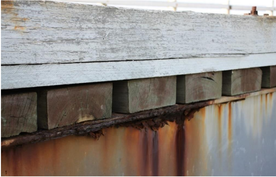
Rusting girders. June 2021
