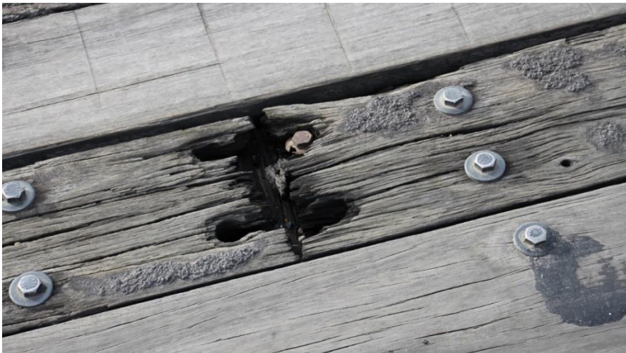
Failing deck timber. This common problem is caused by water entering the timber via the screw holes and causing decay. June 2021.
