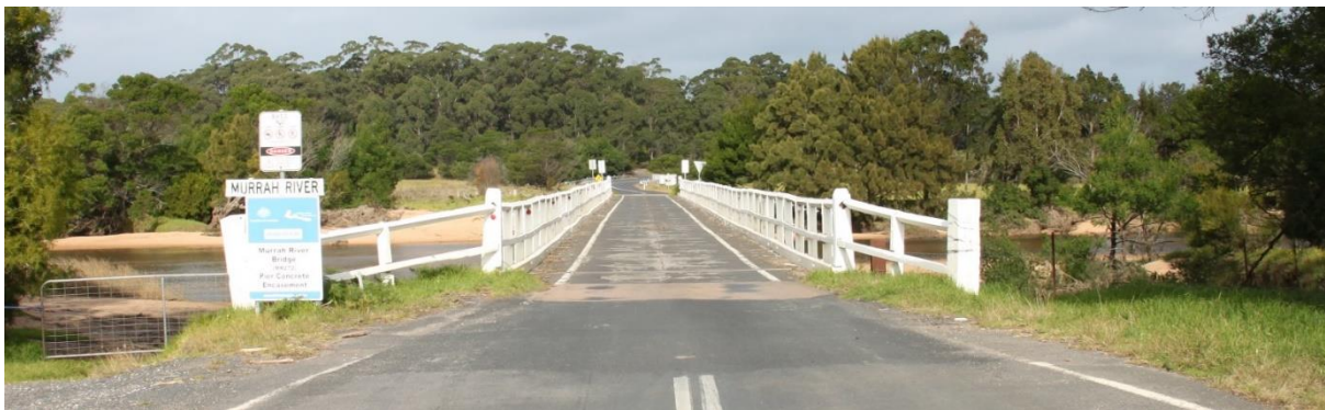
Murrah Bridge 2021. From the tourist perspective the bridge presents as a timber structure.
