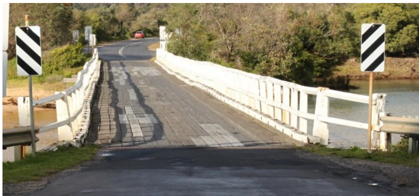
Cuttagee Bridge looking south. The many irregularities in the substructure are reflected in the 'wavy' lines of handrails, kerbing and the deck surface itself. Many timbers have decayed, and metal is rusting. June 2021
