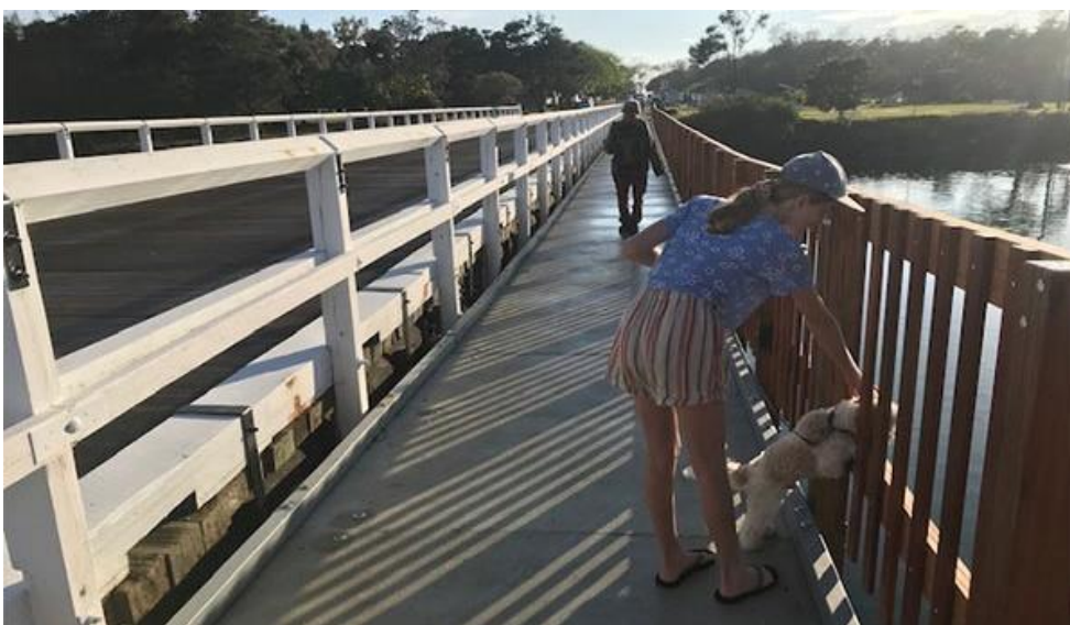
The historic timber railings on the vehicle bridge have been upgraded and painted. The balustrade on the pedestrian bridge has also been upgraded by changing from galvanised steel pipe to clear finished timber.
