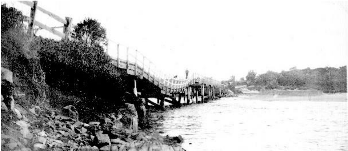
'The piles on the upstream of Cuttagee Bridge were undermined, tipping the bridge sideways so that it could be used only by light traffic using extreme caution'. Looking back: The floods of 1934, Bega District News 23 MARCH 2018.
