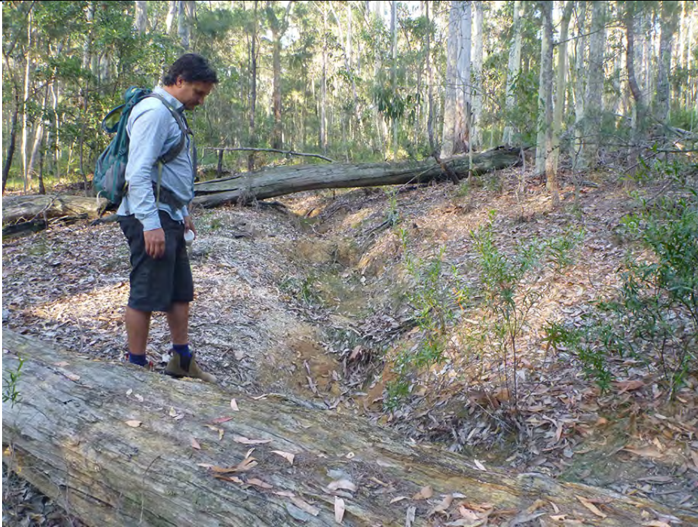
Figure B23 Example of rill erosion on the hill slope of management area 5 caused by disturbance of the soil surface likely due to historical logging operations. This issue can be treated by constructing several log berms to disperse surface runoff, trap sediments and encourage colonisation of vegetation.
