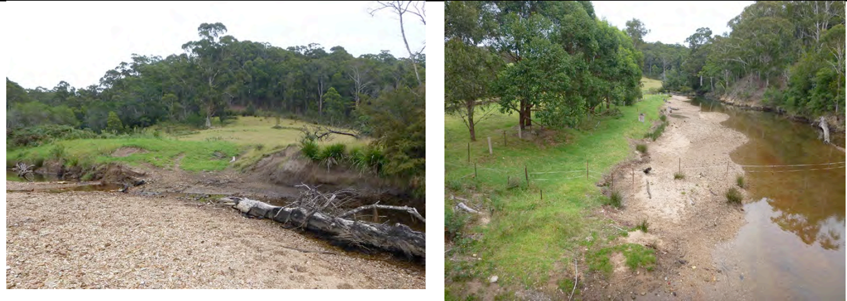
Figure B2 Section of degraded bank where stock cross Nelson Creek to access grazing areas ( left image ). Stock are occasionally provided access the streamside zone and enter Nelson Creek upstream of the Tathra-Bermagui Road bridge ( right image ).
