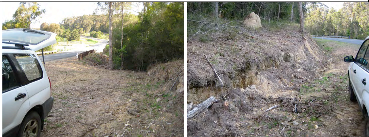
Figure B6 The western side of Tathra-Bermagui Road where surface road runoff drains to Nelson Creek ( left image ). Example of an area of eroding roadside embankment that could be improved through appropriate battering ( right image ).
