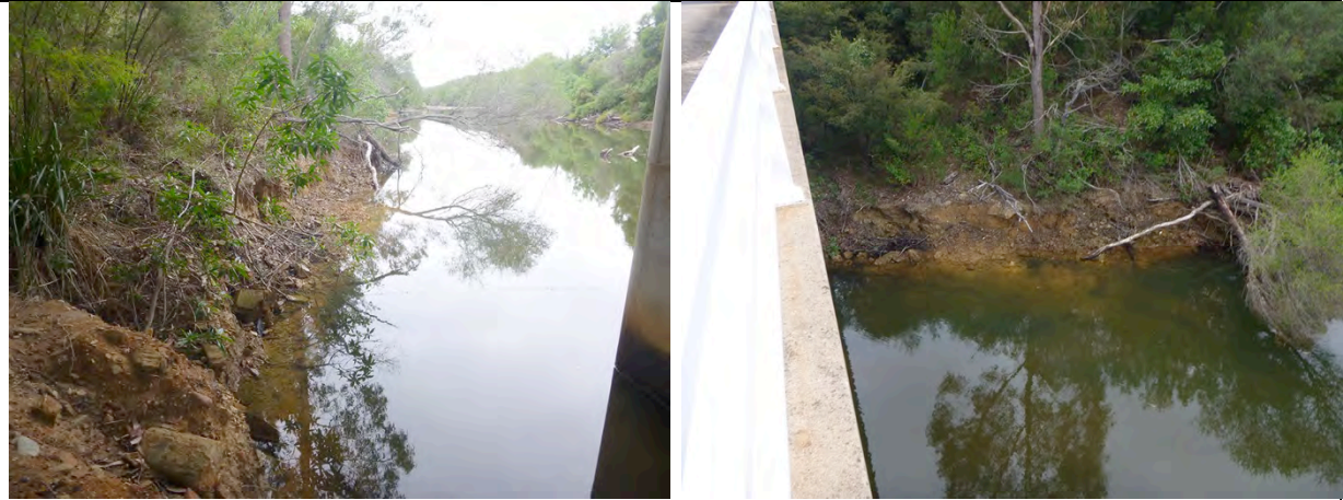
Figure B5 Minor erosion evident to the bridge abutments on the left bank ( left image ). View of erosion to left bank from above ( right image ).
