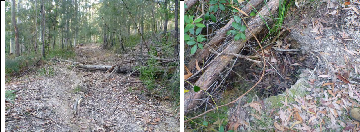
Figure B24 Example of NPWS management track showing minor to moderate erosion ( left image ). Localised areas of road erosion include nick-points with potential to develop into gullies if left unaddressed ( right image ).
