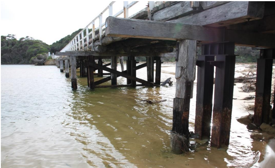
View from South abutment looking north at pier 9. June 2021. Note extended headstocks, introduced steel piers, butt-spliced timber piers and rust at base of steel work.
