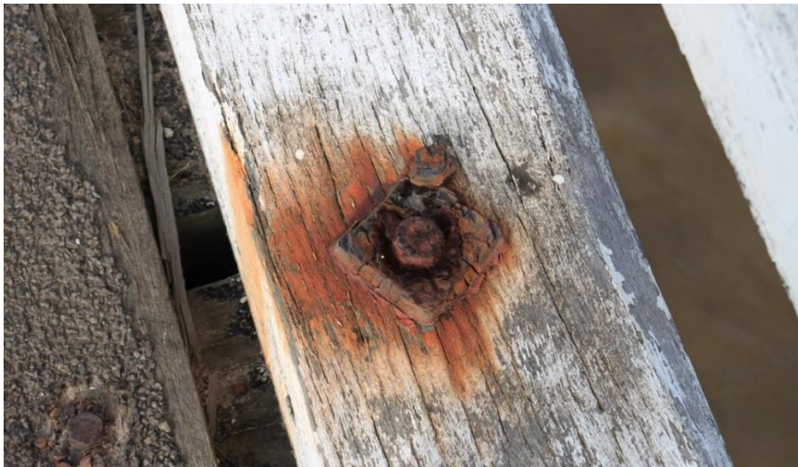
Rusting fixings holding down kerbs, June 2021
