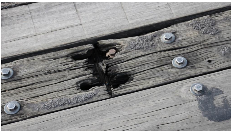
Failing deck timber. This common problem is caused by water entering the timber via the screw holes and causing decay. June 2021.
