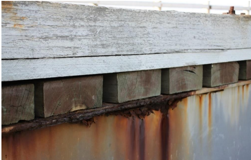
Rusting girders. June 2021
