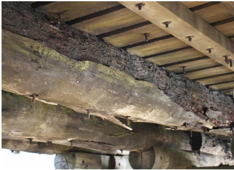
Cuttagee Bridge girders at Span 9, photographed June 2021. The good condition of the underside of decking suggests that timbers were replaced in relatively recent times.
