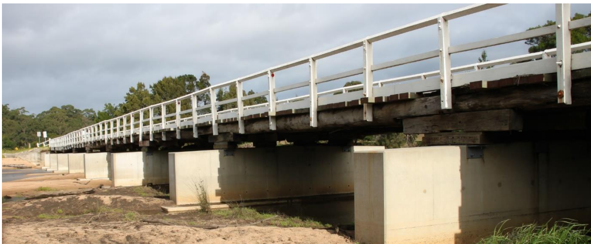
The timber upper structure is supported on relatively recent concrete piers that may be wide enough to support a second lane if the bridge needs to be widened.
