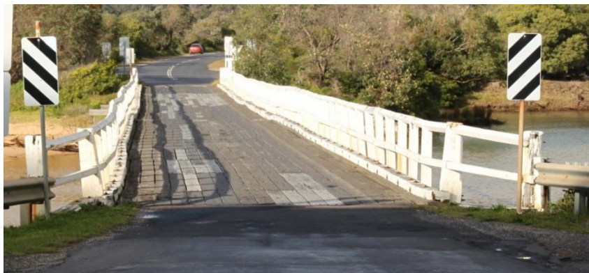
Cuttagee Bridge looking south. The many irregularities in the substructure are reflected in the 'wavy' lines of handrails, kerbing and the deck surface itself. Many timbers have decayed, and metal is rusting. June 2021
