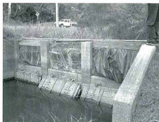
Russell Creek Weir and floodgates, stops brackish estuarine water from backing up into Penooka Swamp.
