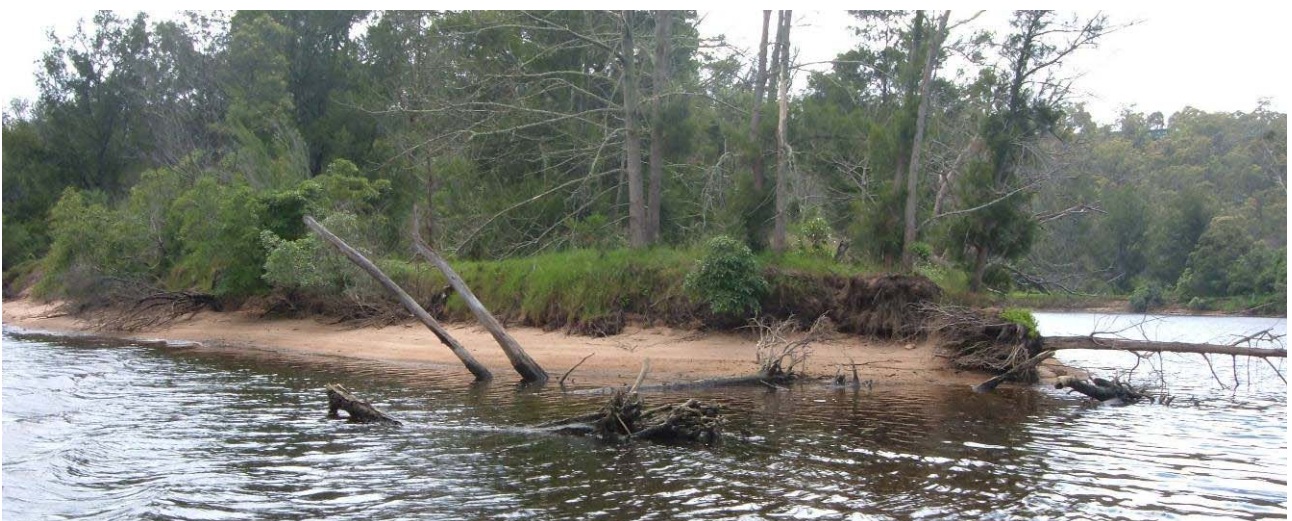
Figure 2-7 Bank Erosion: Site C (refer Figure B-8)
