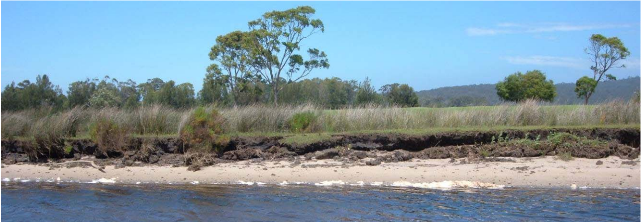
Figure 2-5 Bank Erosion: Site A (refer Figure B-8)
