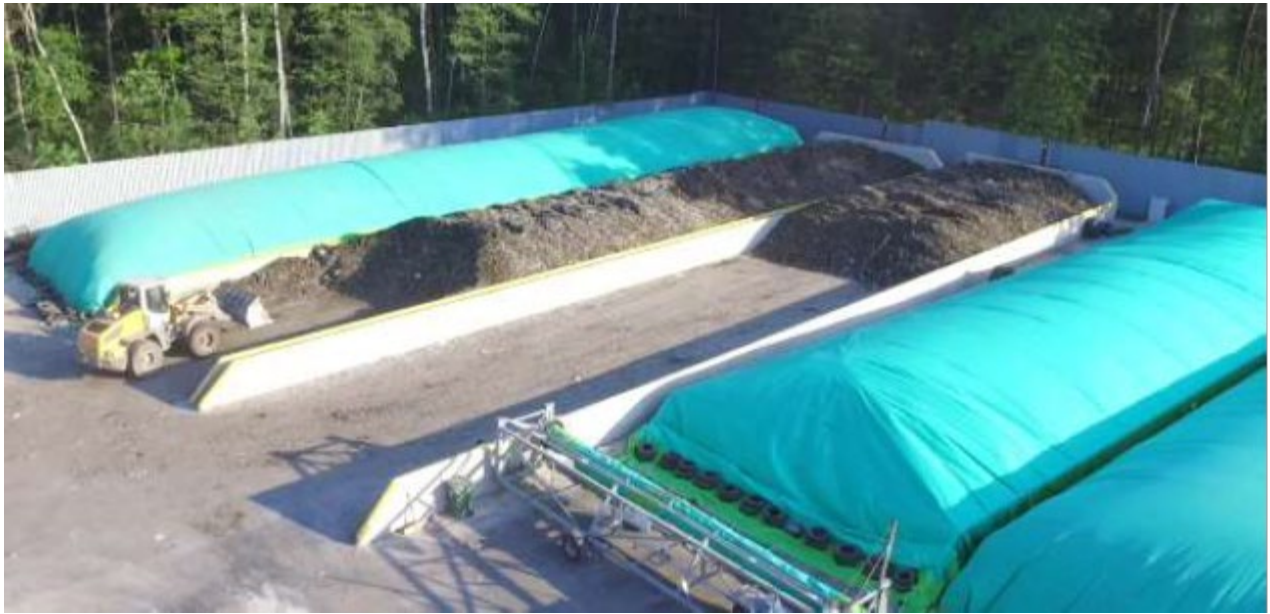
Figure 3 Example CASP bays in operation
