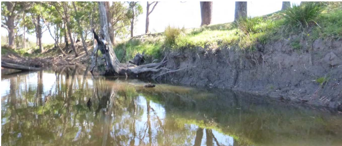
Figure 19. Example of bank toe erosion occurring along lower reach of Sandy Creek.
