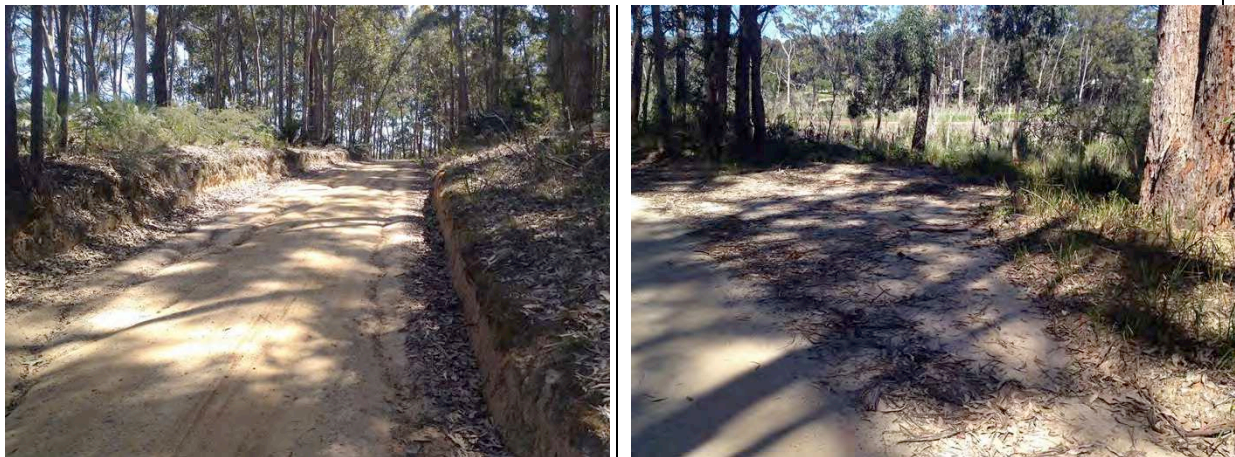
Figure B20 Moderately sloping section of crown road requiring improved surface runoff controls and improved maintenance schedule undertaken in liaison with landholders ( left image ). The mitre drain at the base of the road slope increasing in size with dispersible soil fractions entering the saltmarsh in high rainfall events ( right image ).
