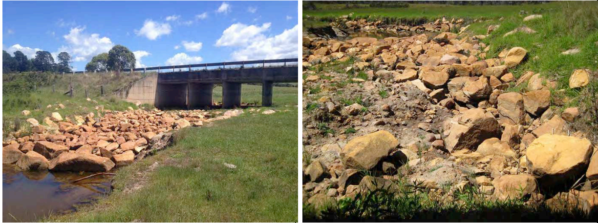
Figure B15 The rock chute outlet below the box-culvert ( left image ). Example of the large boulders comprising the rock chute and disturbance to bed sediments occurring during high flow events ( right image ).
