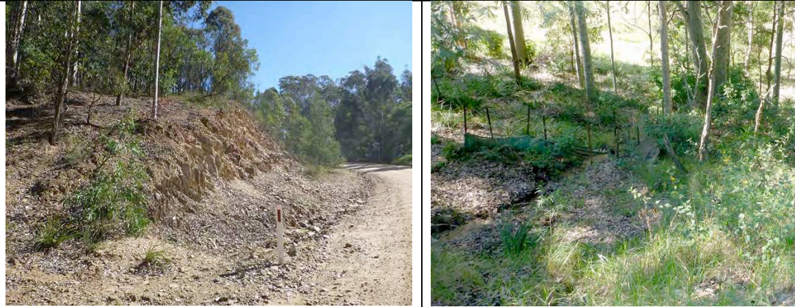
Figure B2 Example of a hillslope and unstable roadside embankment of Dr George Mountain Road that continues to erode and supply dispersible sediment fractions during rainfall events ( left image ). Road surface runoff is directed to the crown road reserve via two stormwater pipes where sediment deposition below pipe outlets is evident. Siltation barrier below one of the pipe outlets is damaged and no longer functional with sediment being delivered further downslope to private land ( right image ).
