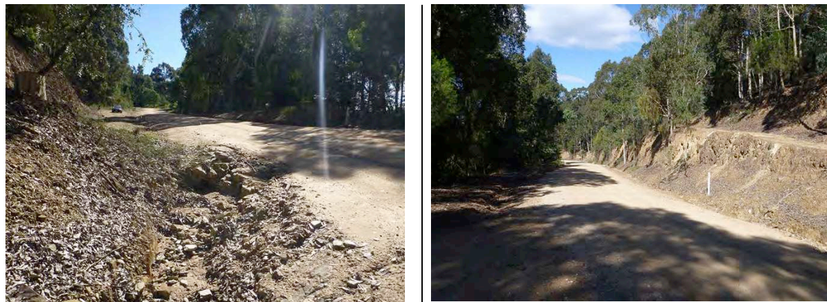
Figure B3 Third storm-water pipe outlet (along the 700m road section) that discharges to roadside drain below embankment ( left image ). From the pipe outlet, road surface runoff flows a further 400m to Tathra-Bermagui Road ( right image ).
