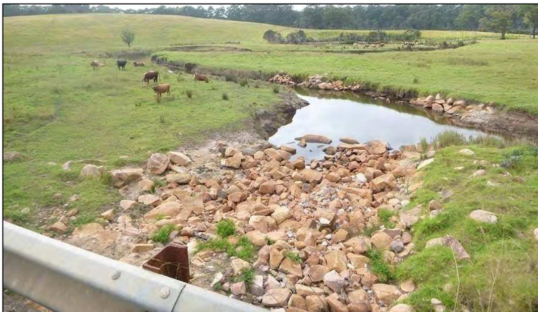
Figure 21. Localised bank erosion occurring adjacent to the rock chute at the box culvert outlet on Booth's Creek.
