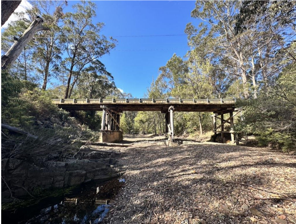
Figure 3-5, Existing bridge from western side showing forest vegetation extent grading into riparian area.
