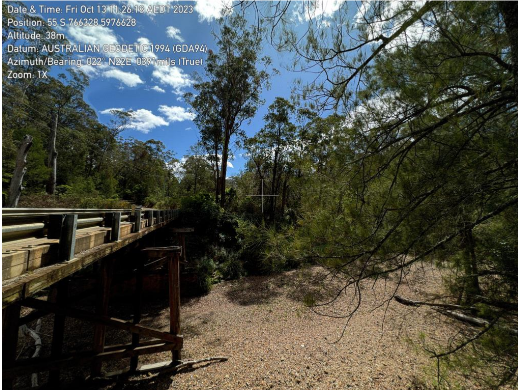
Photo 3, Alignment of proposed bridge facing north, vegetation in middle of image will be removed.
