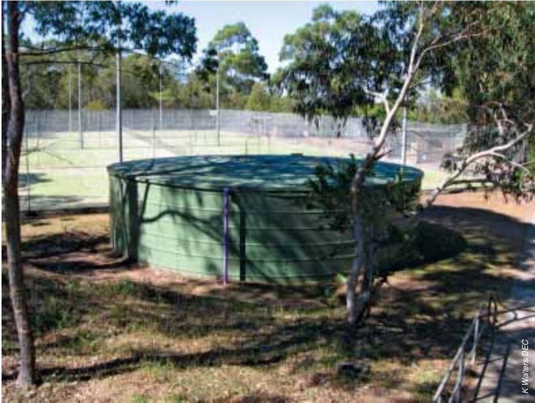
Stormwater storage at Pennant Hills Park stormwater reuse scheme
