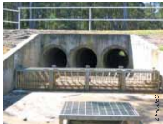
Gross pollutant trap on pipes upstream of the scheme
