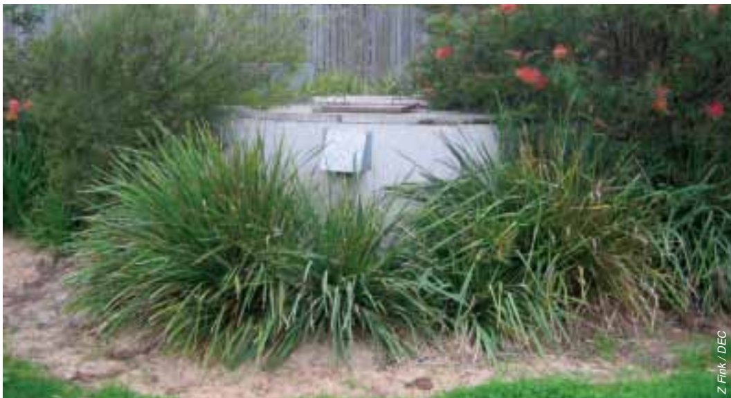
Irrigation storage tank, Powells Creek Park
