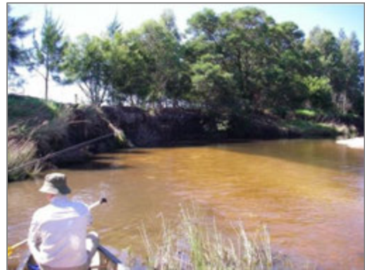
Example of Bank Erosion in Pambula Estuary (SRCMA, 2012)
