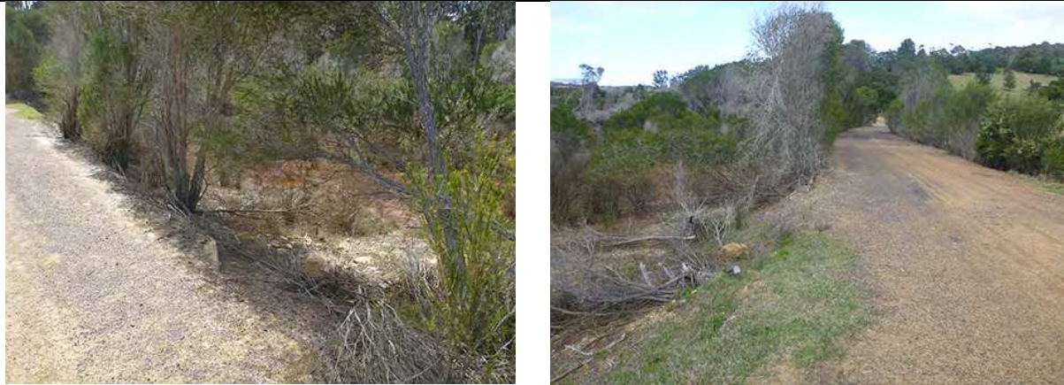
Figure B10 Examples of localised minor erosion points on the eastern side of roadside embankment.
