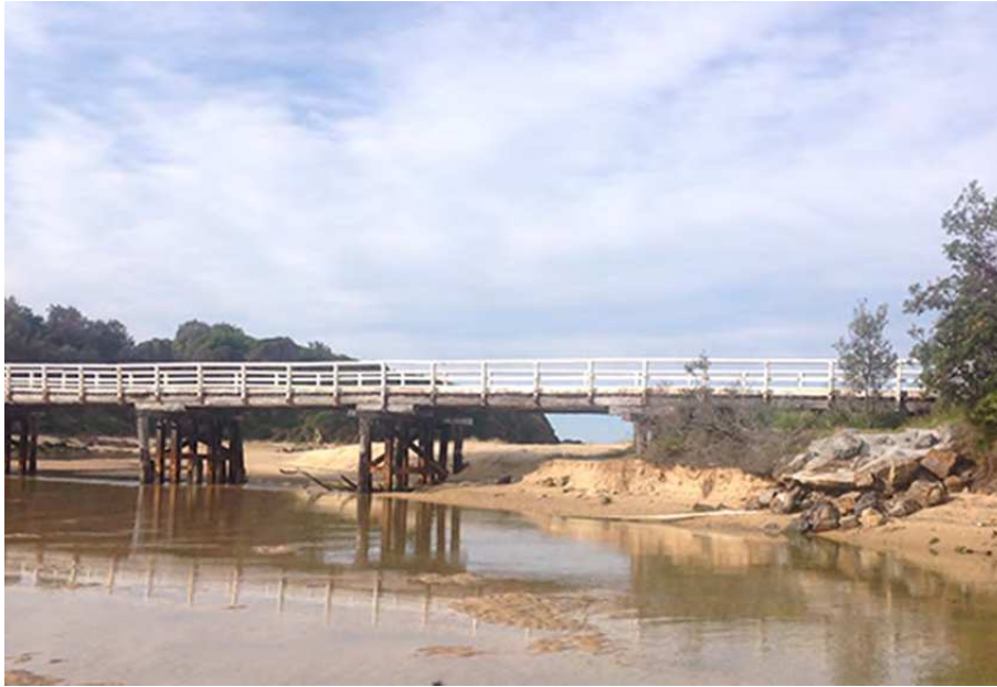
Figure B25 Recent bed erosion around the foundations and support poles of the Tathra-Bermagui Road bridge with potential to threaten the structural integrity of bridge.
