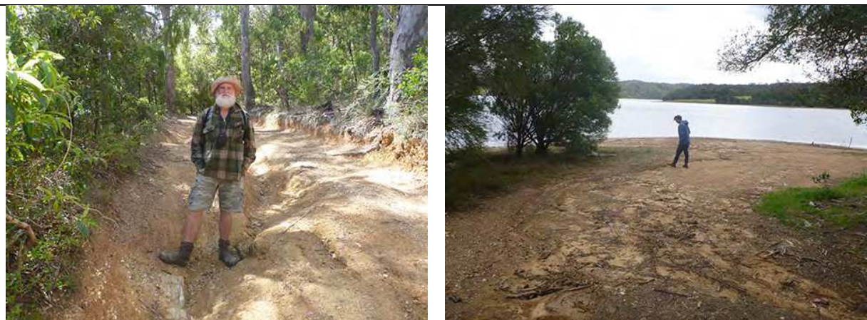
Figure B2 Crown access road with example of section with deep rutting due to inadequate stormwater runoff controls ( left image ). Ongoing road erosion is contributing sediment fines to the estuary foreshore with potential impacts to adjacent nearby seagrass community ( right image ).
