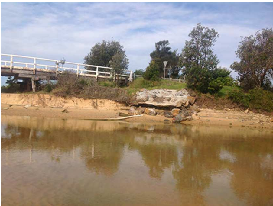
Figure B24 Community access to estuary foreshore degraded following recent erosion.
