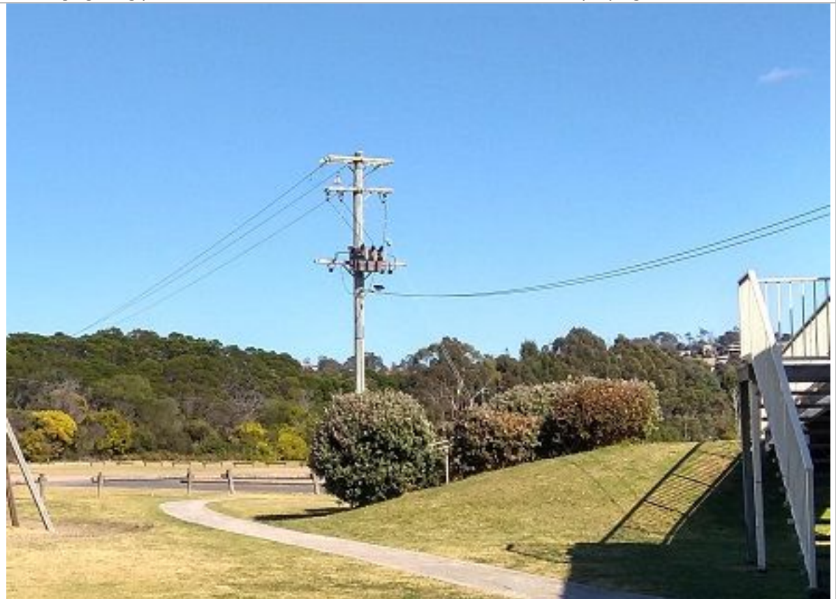
Current power connection to be upgraded to new sub-station.
