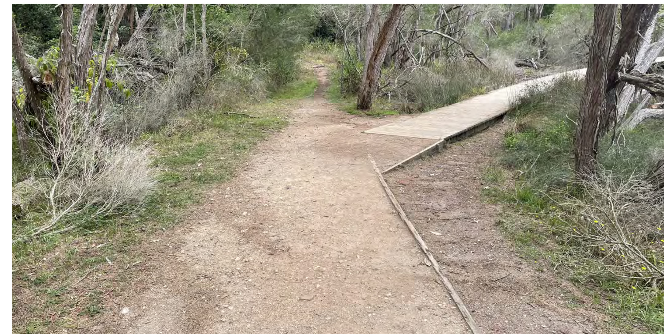
While in urgent need of repair, the character will be inspired by the existing with far better accessibility, durability and high quality finished. The clarity of wayfinding will be improved.
