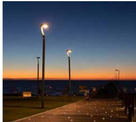
Overhead luminaires at entry node
