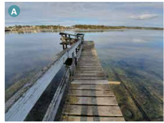
THE EXISTING JETTY IS IN AN EXCELLENT LOCATION AND IS PERFECT FOR SWIMMING, HOWEVER IT'S GETTING RICKETY AND RUN DOWN. THE CONCEPT PROPOSES TO ENHANCE THIS JETTY TO PROVIDE A WIDER, MORE ACCESSIBLE APPROACH AND LARGER PLATFORM FOR SWIMMING AND FISHING. THE LADDER FOR ENTRY/EXIT IS PROPOSED TO BE RETAINED FOR THOSE WANTING TO SWIM.
