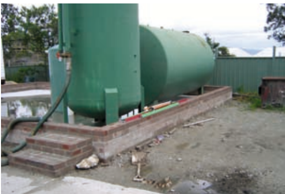
Above: Procedures need to be put in place to manage water that accumulates in unroofed secondary containment areas
