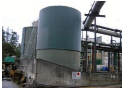
Above: Shielding can be installed where the secondary containment area is insufficient to contain leaks from the top half of the tank.
