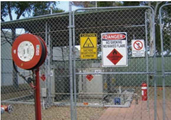
Below: This secondary containment area is roofed, has a sunken concrete bund, appropriate signage and an electronic alarm system.
