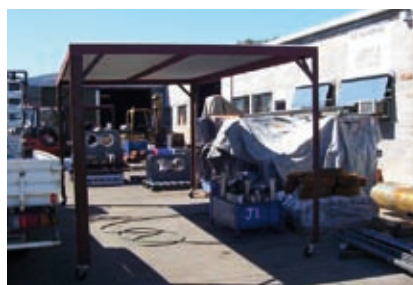
Above: Roofs keep rainwater out of secondary containment areas but can restrict access. This portable roof keeps the area dry but can be moved during delivery or despatch.
