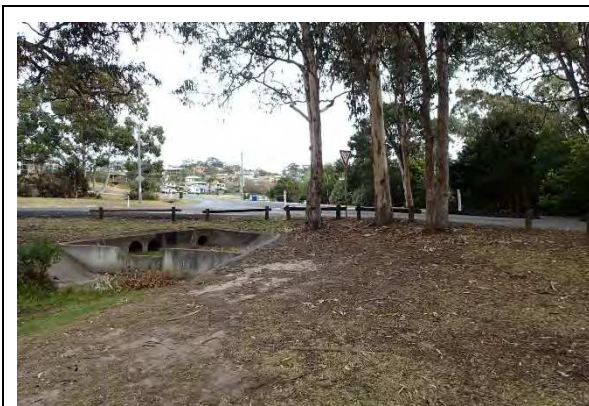
Plate 9. View west to road intersection showing built up roadway and underground stormwater drainage structures.
