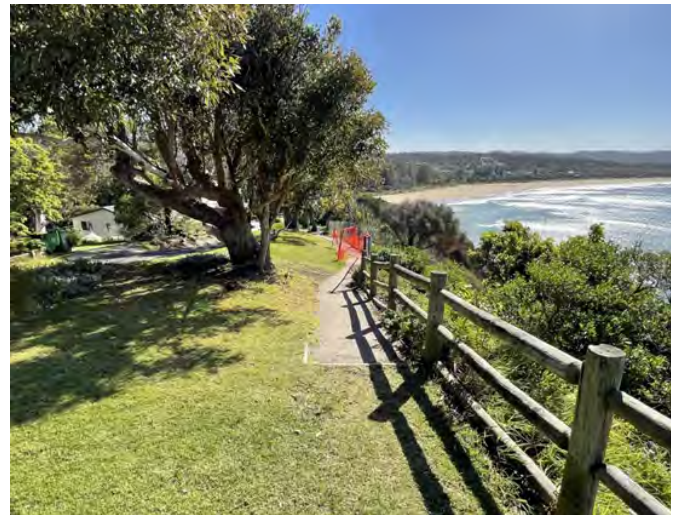
The path is not connected back to the network, and conditions are failing.
